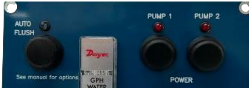
Figure 26: Operator Control Panel Detail
